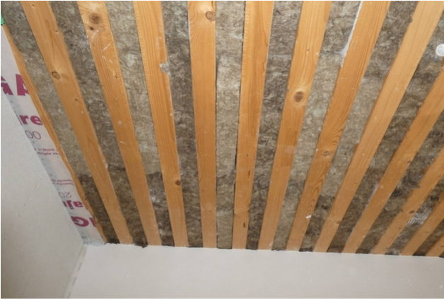
Ceiling insulation in barn conversion
