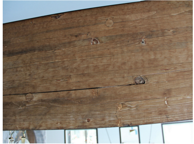
Failure of glulam beams
